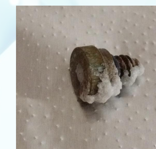
Salt buildup on mister
